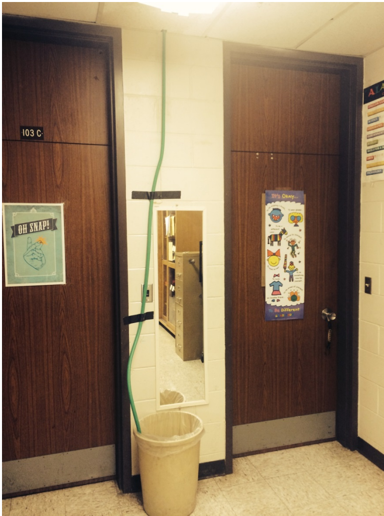
Kenai Middle Leaky Roof
